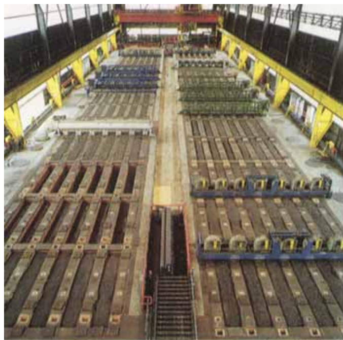
Figure 18: Anode bake furnace in operation
