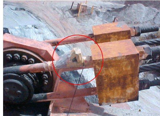
Sensor at one tie beam
